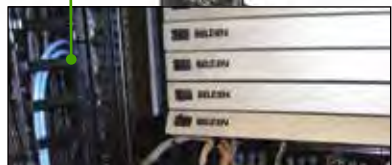
Vertical Manager shown in cabinet
