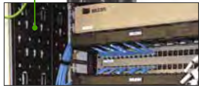
Lacing Panel shown in cabinet
