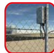
Perimeter Intrusion Detection
