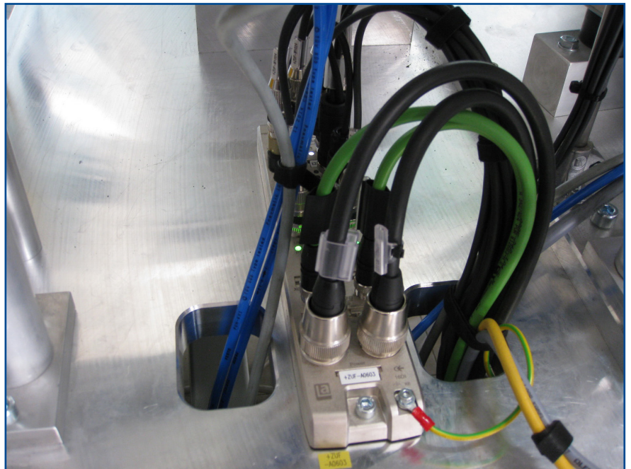
LiON-R module signals from connected sensors and actuators are sent to the controller via one PROFINET data line.
