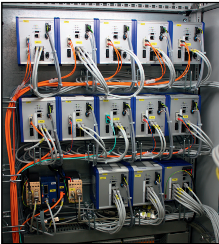
Hirschmann Industrial Ethernet Switches in a Substation
