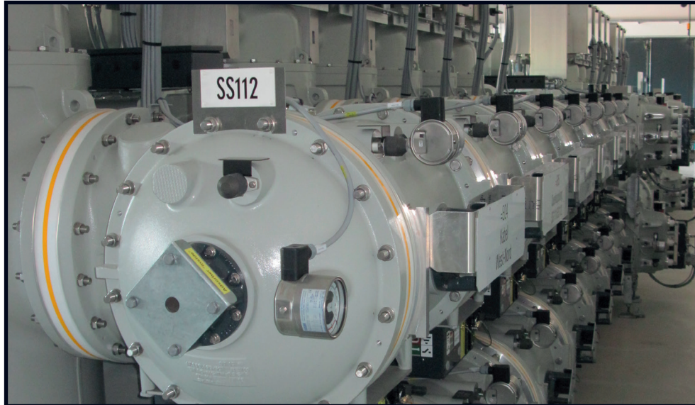
Karlsruhe Needed to Upgrade Its Power Grid
